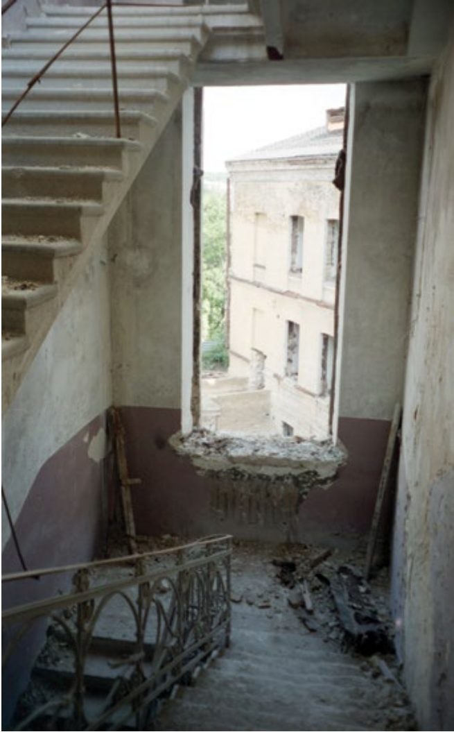
A door on a landing once opened out onto a verandah which had long ago collapsed. Often servants slept on pallets under stairs such as these.
